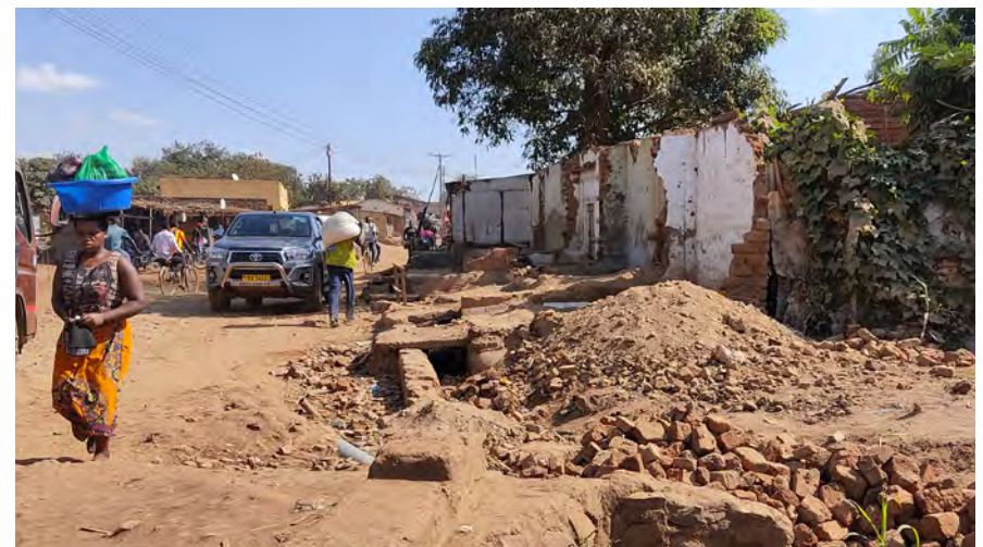
Figure 1 Some of the Police Houses being constructed at Area 30 Police Headquarters in Lilongwe, Malawi www.africa-press.net/malawi/all-news/police-houses-change-the-face-of-jenda-rural-growth-centre (2022)
